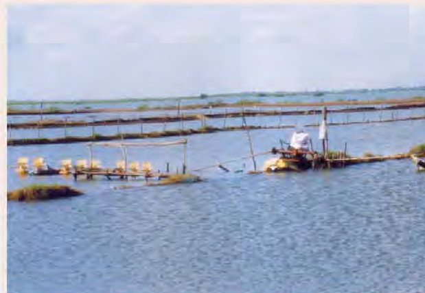
Damage to shrimp pond bunds due to Nisha
