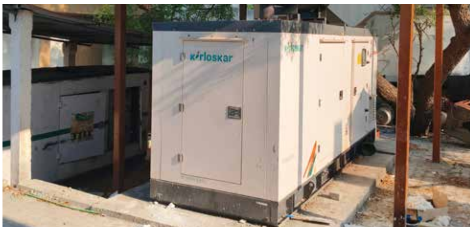
Generator facility for hatchery
