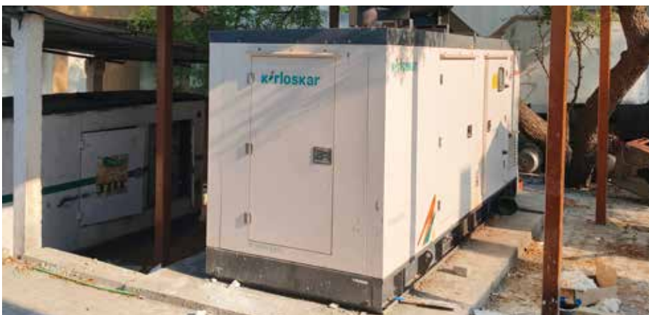
Generator facility for hatchery
